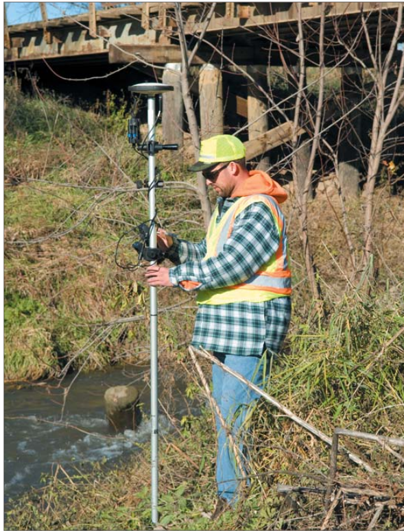
Ten years ago it took a four-person crew five days to do a bridge replacement survey. Today, it takes one person one day to complete the same task.
