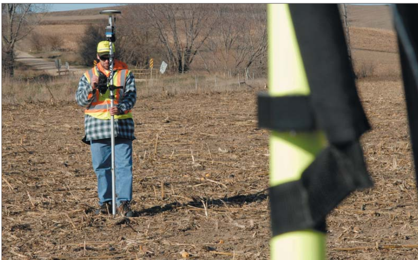
Only one field technician is required to collect real-time, centimeter-accurate survey points for a bridge replacement project.
