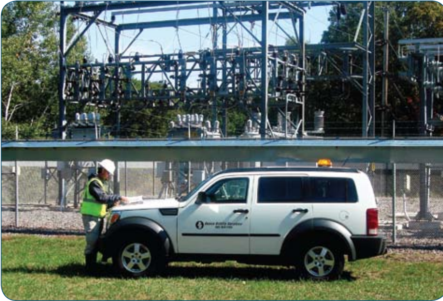
Fig. 3: Working individually circuit by circuit, Hance field technicians collect data at a substation.
