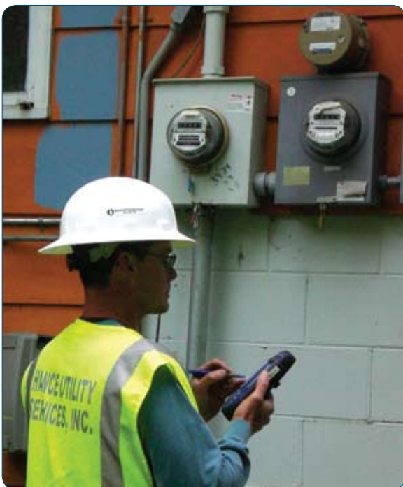
Fig. 1: Hance Utility Services field technician collects data at a customer meter.
